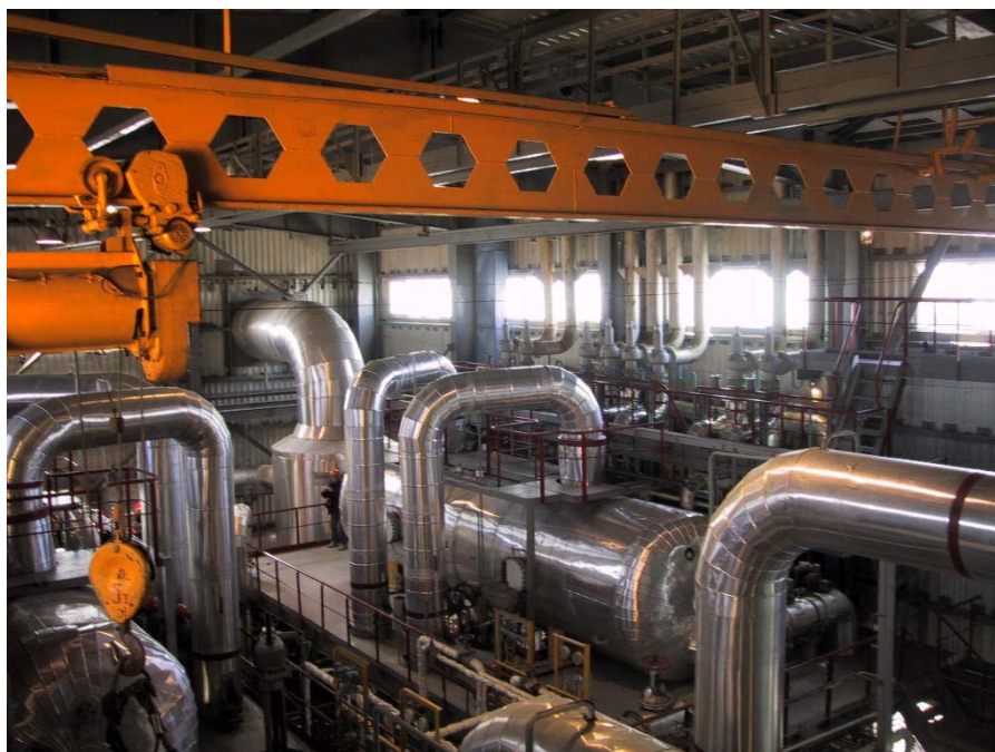
Figure 4,b. Mutnovsky geothermal power plant (MGeoPP). Primary separators provide MGeoPP with the high-quality steam. Photo of Svalova V.B.
