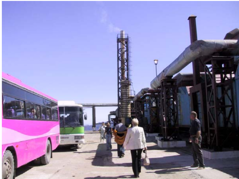
Figure 3,a. Verkhne-Mutnovsky geothermal power plant (GeoPP). First ecologically clean GeoPP. Photo of Svalova V.B.
